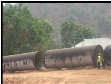
Plate III. The 75 Km Long, 3m Inner Diameter Transfer Pipes
