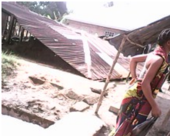
Plate 6. Collapsed building as a result of flood
